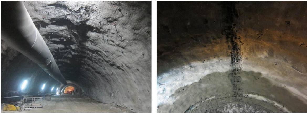
Fig. 2. Shearing of lining due to localized shearing along foliation (left), and open slot in the lining to allow for localized displacements without damage to the lining.
