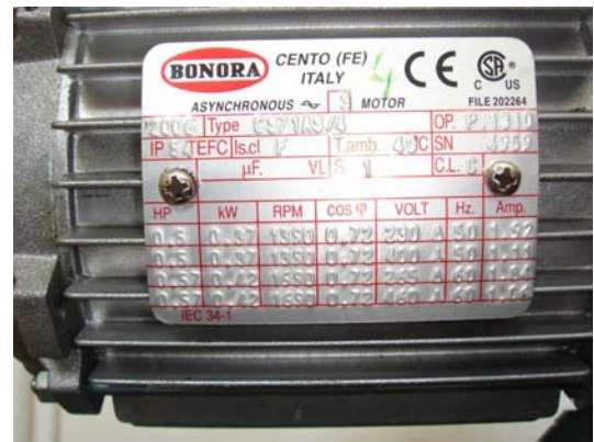
Figure 4.31: Identification Plate (Induction Motor)
