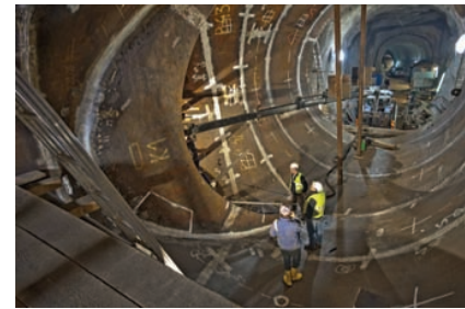
Figure 1: Erection state of the bifurcator of Limberg II pumped storage project, developed by Verbund Hydro Power AG, Austria (main diameter 7.6m, HSS of grade S550QL)
