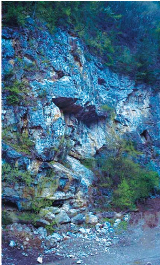
Fig. 1 Small block failure in a road cut formed by a cross joint intersecting a major joint.
