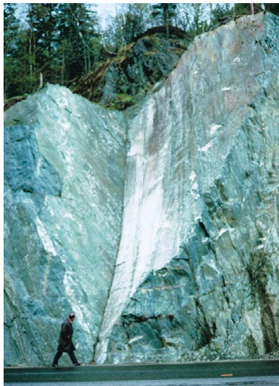
Fig. 3 Wedge failure in a foliated rock mass. Note the curved line of intersection indicating non-planar joint surfaces.
