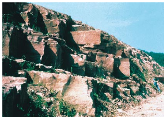
Fig. 9 Photo of a failing rock cut showing the original slope height and approximate angle. Note the shallow dipping claystone beds forming the breaks in the slope.
