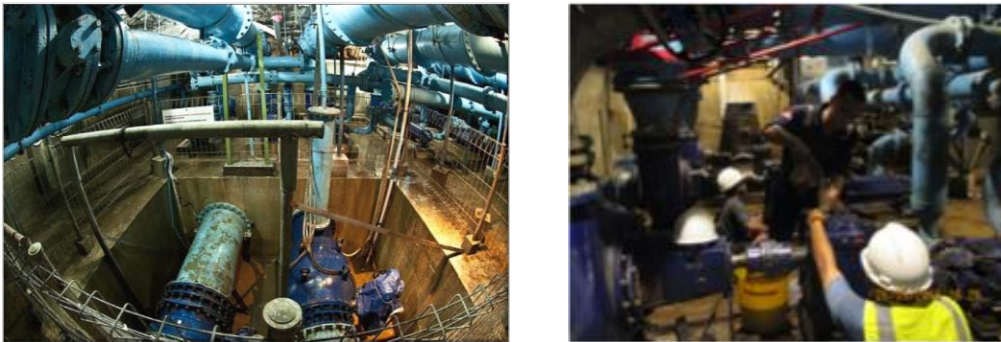
Fig. 3 The condition of Bribin in 2012-left (10) and 2016-right (BBWS SO documentation)
