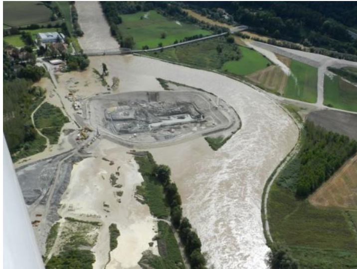
Fig. 8: Photograph of the construction pit site and the diversion channel during high water in September 2014 (discharge approx. 2000 m 3 /s) (source: 24ur.com).
