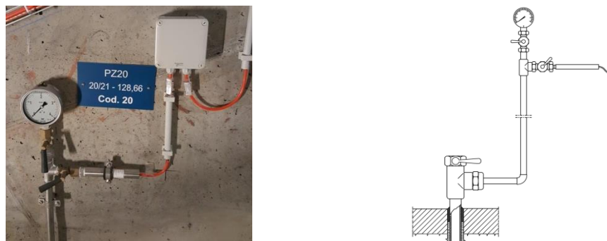
Fig. 3 Piezometer with automated readings.
