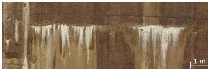
Fig 5: Ortho image of a defect region on the downstream side of the Drossen dam (block 16), derived from 21 OAC textures (1 pixel corresponds to 2 mm on the surface)
