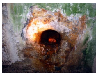
(b) Borehole and the broken tendon remained
