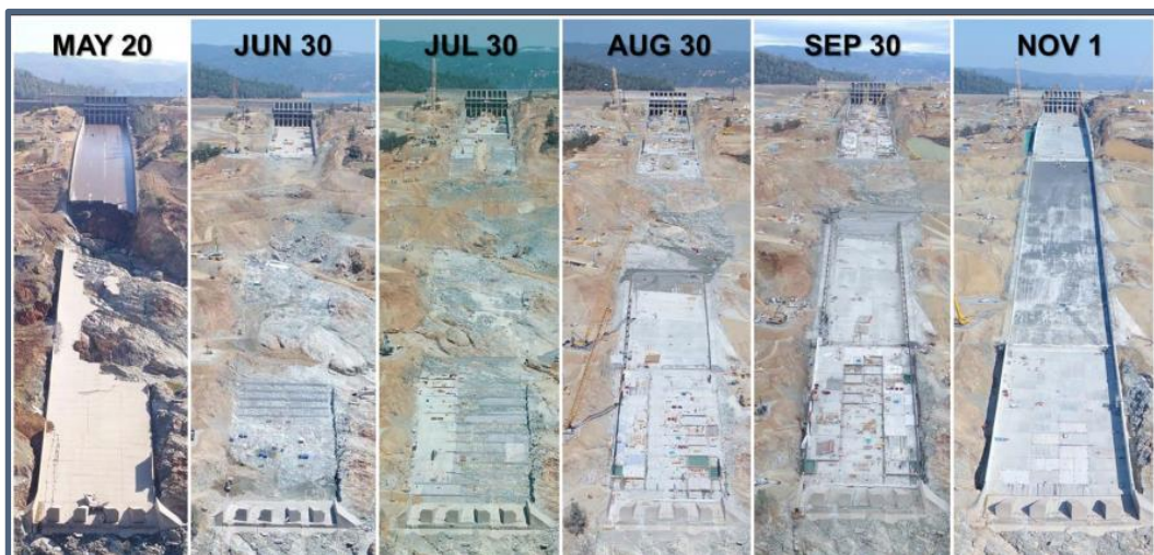
Fig. 10 Aerial views of construction on FCO Spillway chute between May and November 2017
