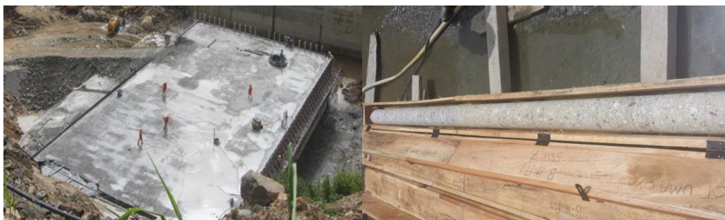
Fig. 6 Curing of RCC lift surface and Core of RCC- length 3m (Uma Oya Project)
