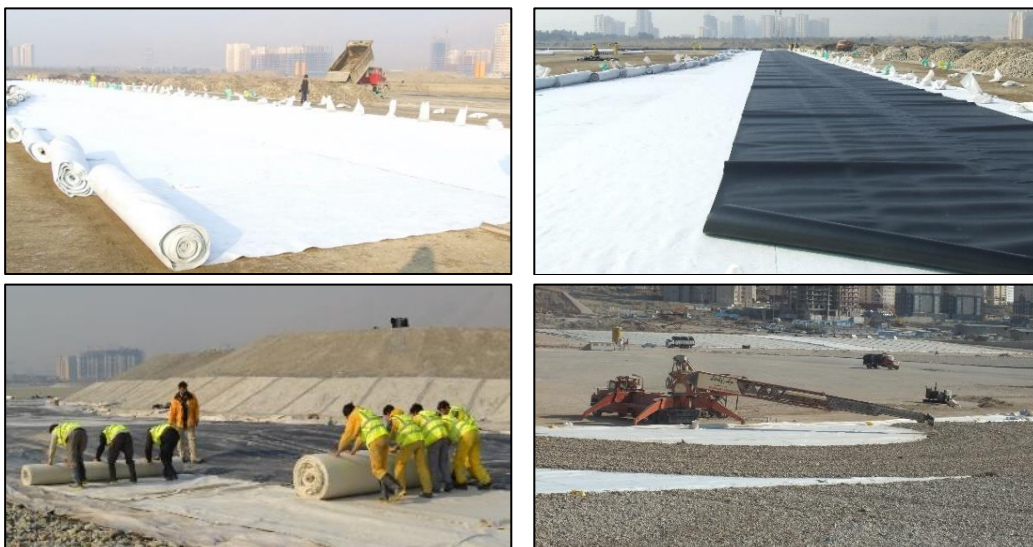
Figure 5. Preparation and Installation Stages for Water tightening of the Chitgar Lake bed
