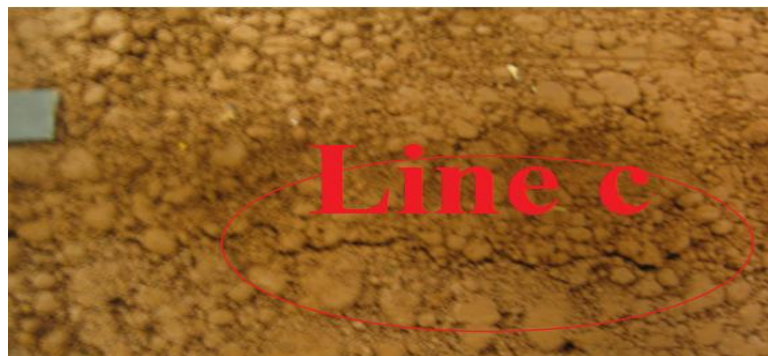
Figure 14: Longitudinal crack at line-c
