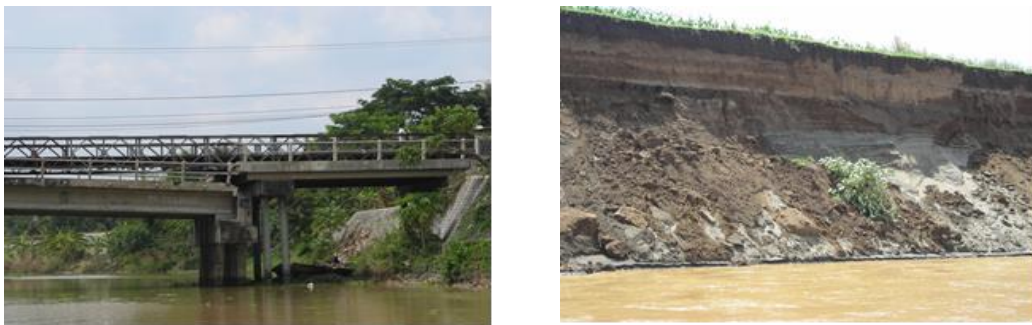
Fig. 2 Damage of Deformation of Bridge Pier and Landslide of Embankment
