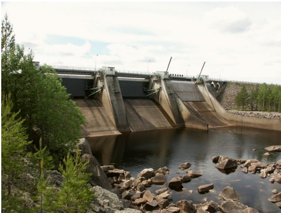
Figure 2: Downstream view of the spillway at Långströmmen prior to dam safety upgrades (Norconsult, 2014).
