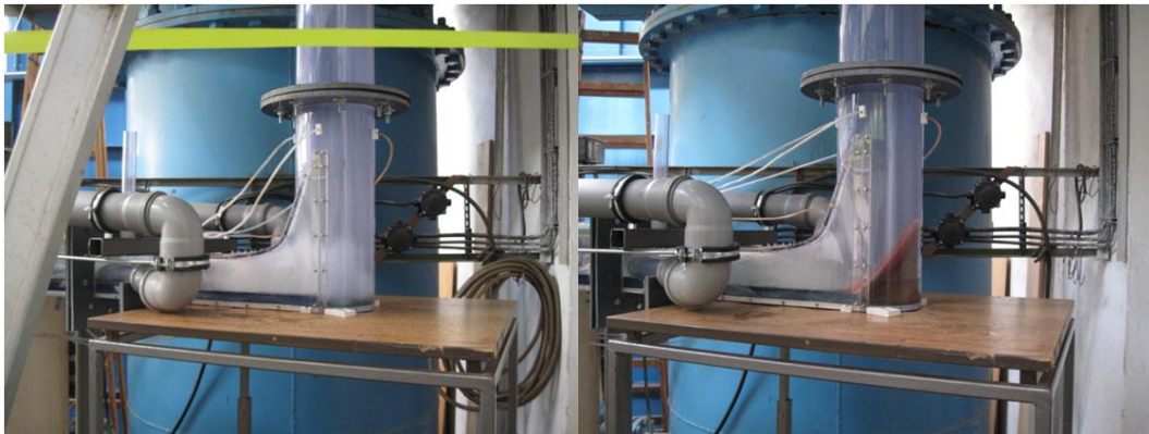
Fig. 4 Rounded bottom end of the vertical shaft Existing design ( Q_{10} ) Updated design ( Q_{10} )
