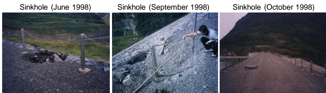
Fig. 2 WM dam sinkhole incidents
