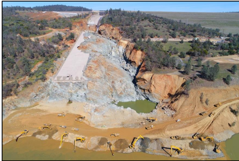
Fig. 10 Ultimate damage at the service spillway
