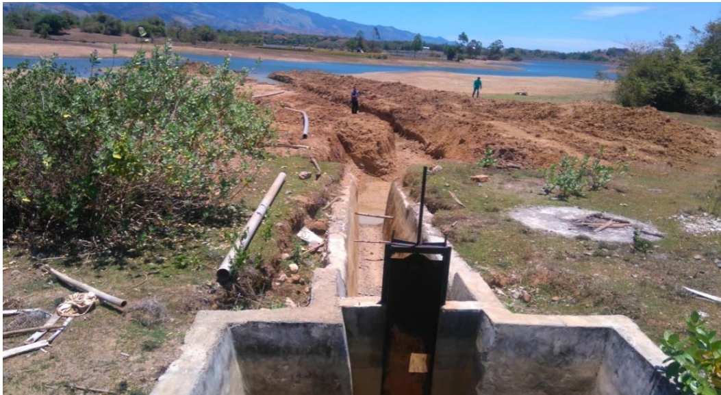
Fig. 3. The Water Siphoning Activities by the Community
