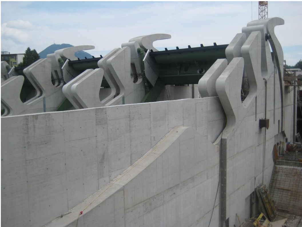
Figure 11: Hydro power plant Lehen, Austria
