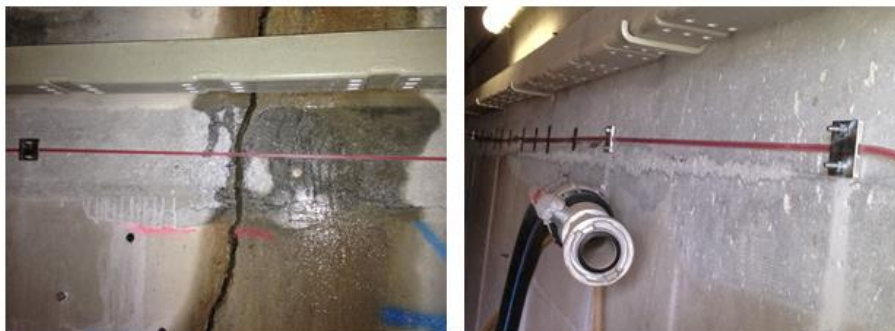
Fig. 11 Strain sensing cable installation on penstock access tunnel
