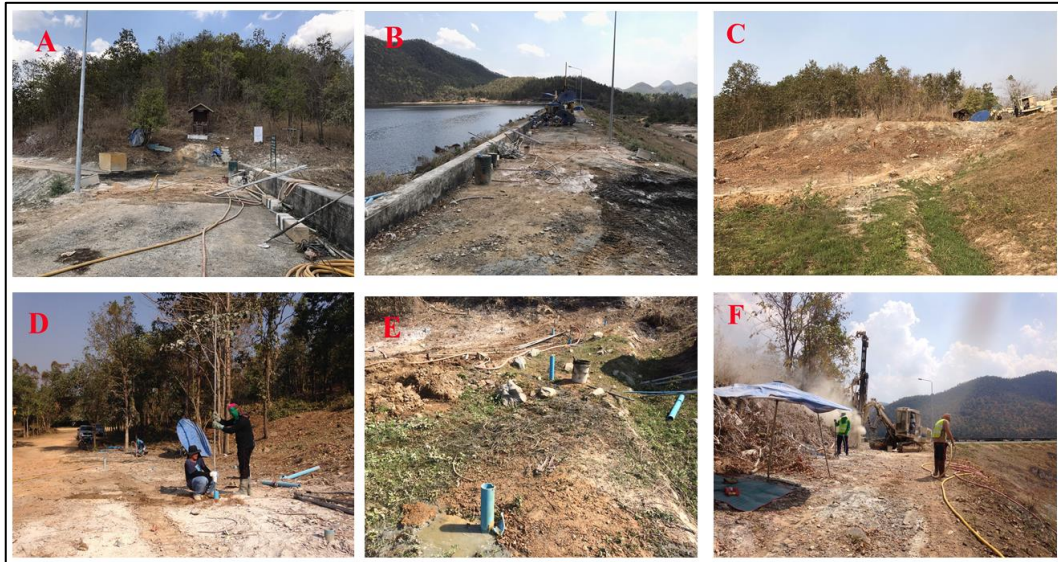
Fig. 7 The working areas as A. Zone C, B. Zone A, B C. Gutting Drain, D. Connection Zone between Abutment and Dam Body, E. Gutting Drain and F. Right Abutment Access Road
