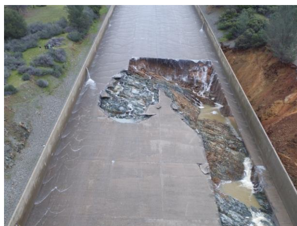
Fig. 3 – Damage to FCO Spillway chute on February 7, 2017
