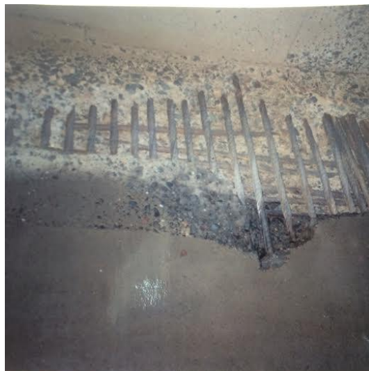
Figure 4. Prototype photograph showing exposed reinforcement inside Tunnel due to cavitations
