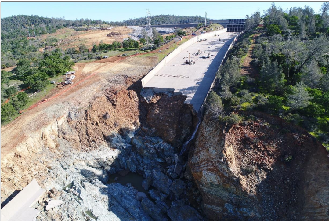
Figure 5 - Photo of the scour hole and channel forming to the left of the FCO Spillway chute illustrating the geology left behind by erosion and scour. Five drill
