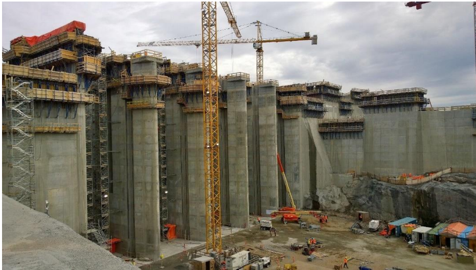
Figure 12: Hydro power plant Muskrat Falls, Canada
