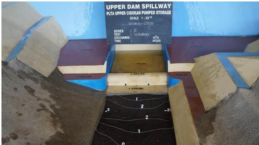
Fig. 9. Scouring condition at downstream of spillway (Scenario 1)
