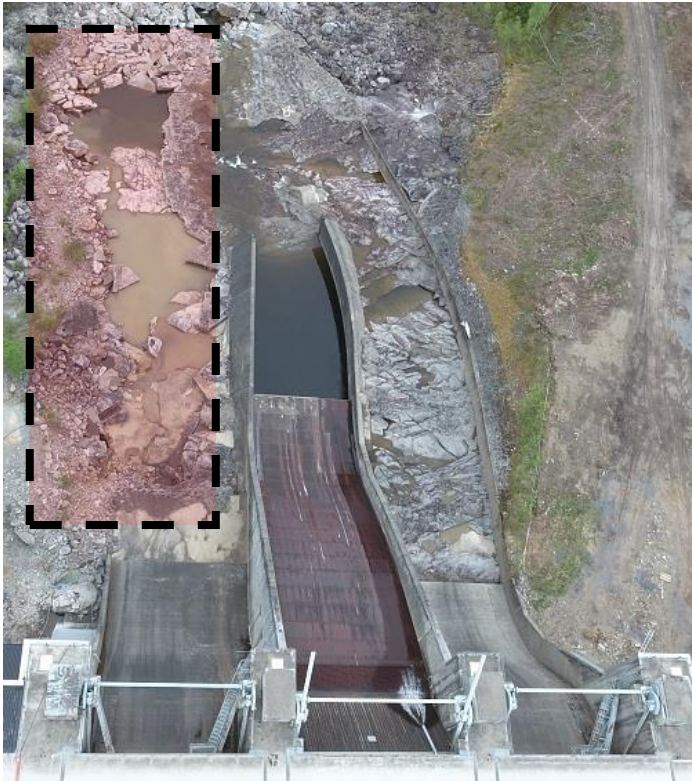
Figure 4 Eroded area (marked red) downstream of the left chute at Ramsele (Norconsult, 2014).
