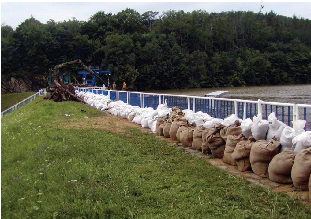
Fig. 6 Sandbags located at the crest of the dam Znojmo to reduce risk of overtopping
