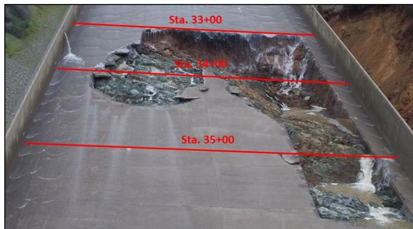
Fig. 9 Service spillway chute damage observed after gates were closed on February 7
