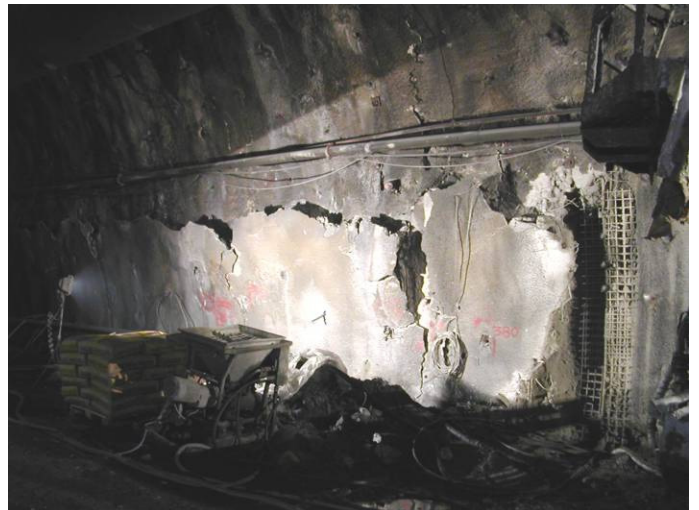
Figure 1. Damaged lining after excessive displacements and exceeded deformability of the shotcrete.
