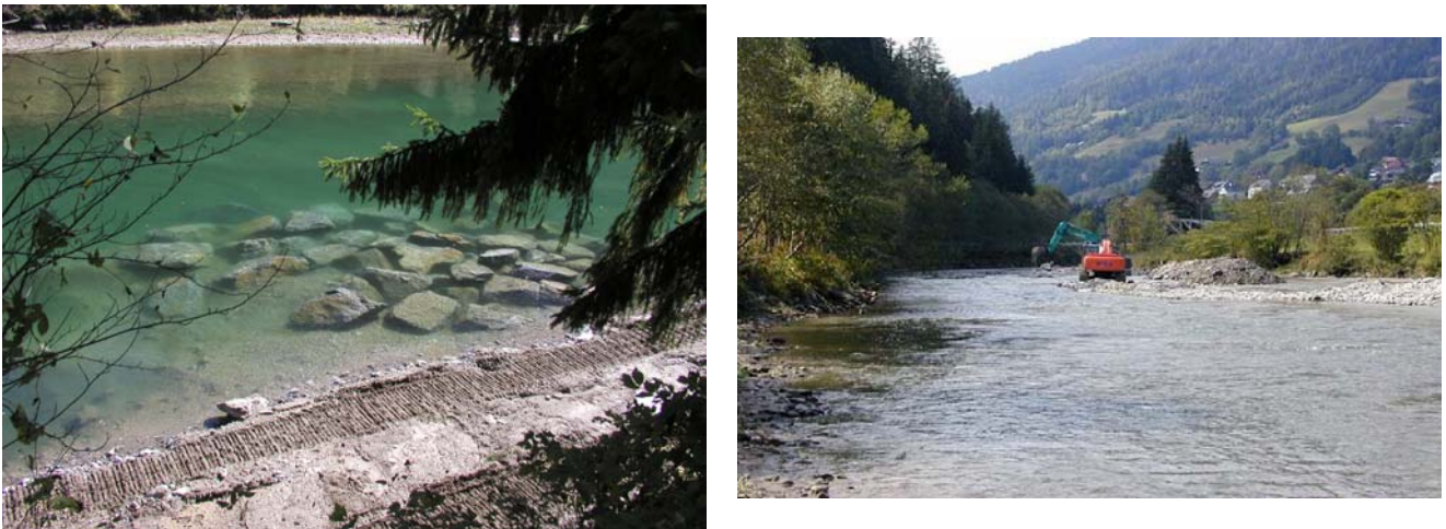
Figure 3 Short groin at the upstream part of the reservoir, excavation of the flushing channel in 2003
