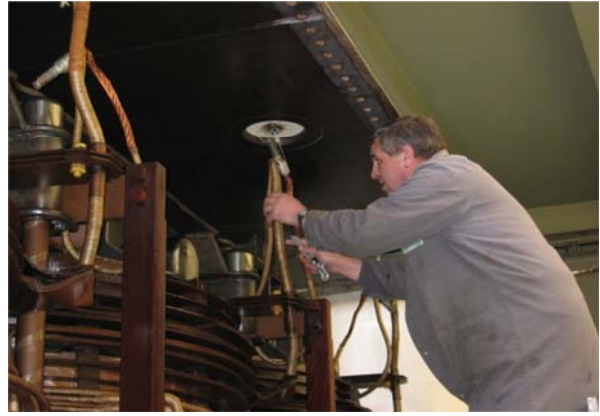
Figure 1: Extraction of a cellulose sample at the connection of the transformer bushings [1]
