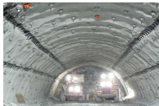
Figure 8. Top heading at the second tube of the Tauertunnel with four rows of ductile elements integrated in the shotcrete lining. Photo: Vergeiner
