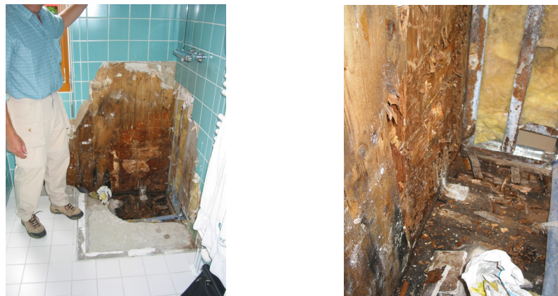
Fig. 18 Damage of the CLT bearing structure caused by moisture ingress in a wet room
