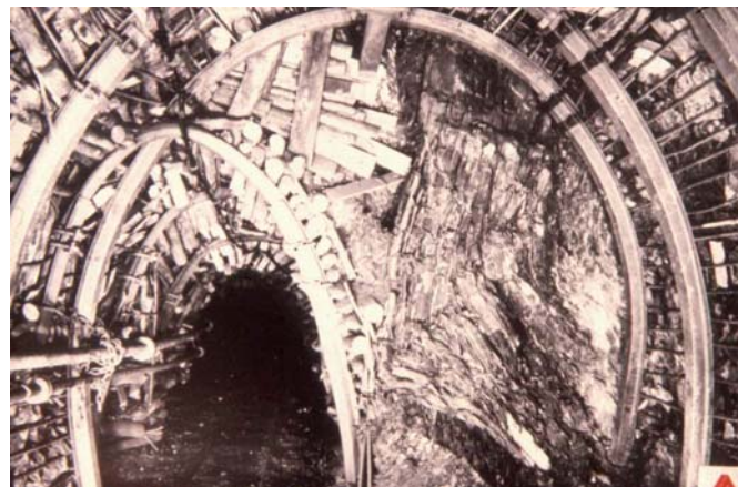
Figure 1. Destroyed steel set support with sliding couplings. Photo: DMT
