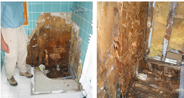
Figure 2: Damage of the CLT bearing structure caused by moisture ingress in a wet room
