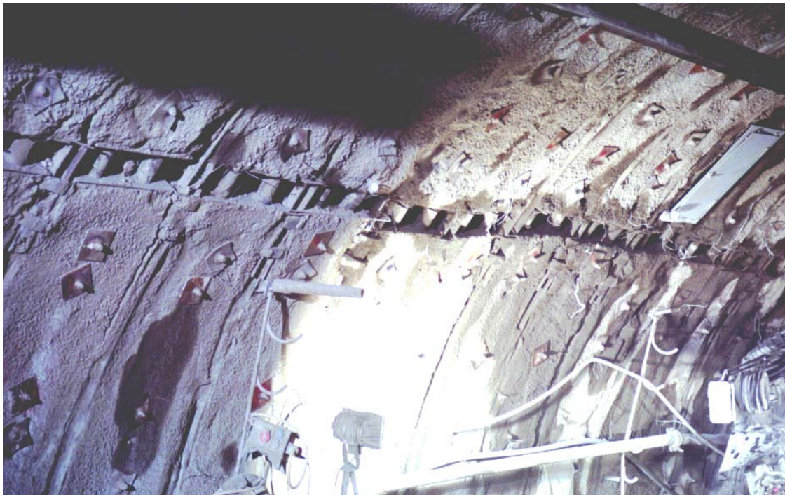
Figure 16: “Semmering” railway tunnel / Austria; improved support system with 150 mm deformed “Lining Stress Controllers” between the lining “segments”
