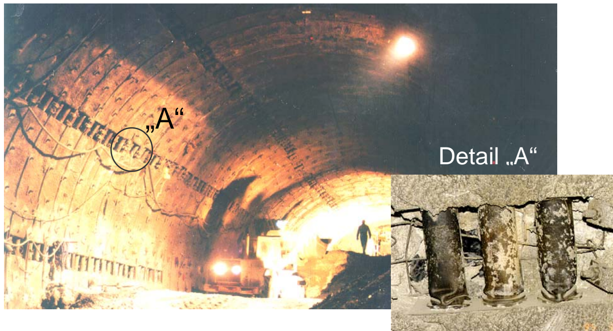
Figure 2: “Haberl Fault”-“Galgenbergtunnel” / Austria; Yielding-steel-elements integrated in deformation gaps of the shotcrete lining [7]
