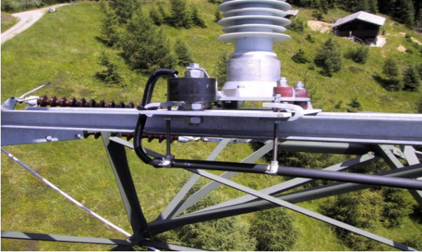
Fig. 9: Arrestor Discharge Logger (SIEMENS) at the line arrestor on the pole arm
