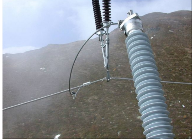
Fig. 7: Line arrester and disconnection device between the phase conductor and the arrester
