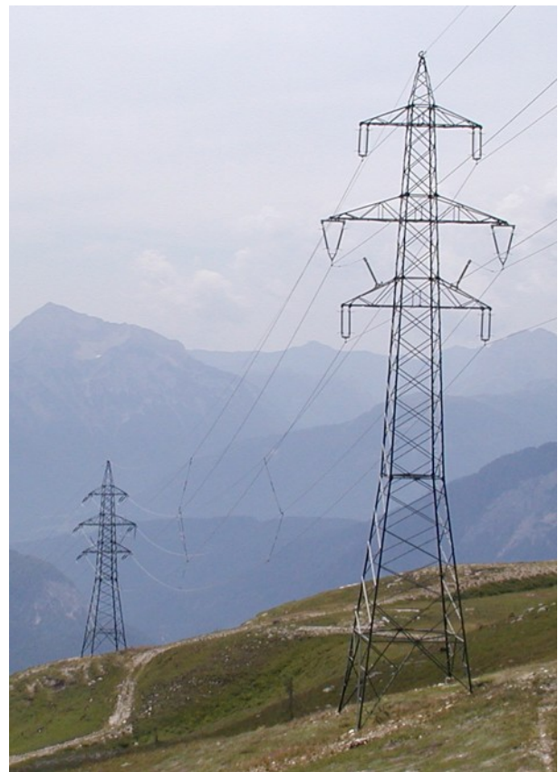
Fig.1: Line arrestor application on a KELAG 110 kV overhead line in this extreme alpine region
