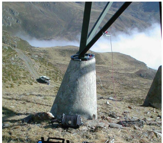
Fig. 8: On site measurements to evaluate the tower grounding situation in the observed line section
