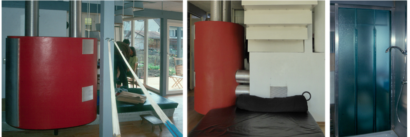
Fig 10 left and center: elliptic hypocaust stove with 'activity bed' in living room right: translucent hypocaust wall in bathroom, made in profile glass, water resistant and used as towel dryer
