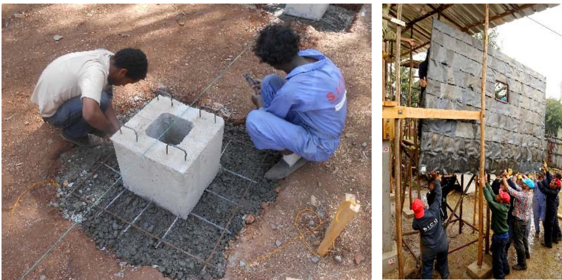
Fig. 5 SICU – placing the prefab foundation (first day) and prefab cladding elements (sixth day)
