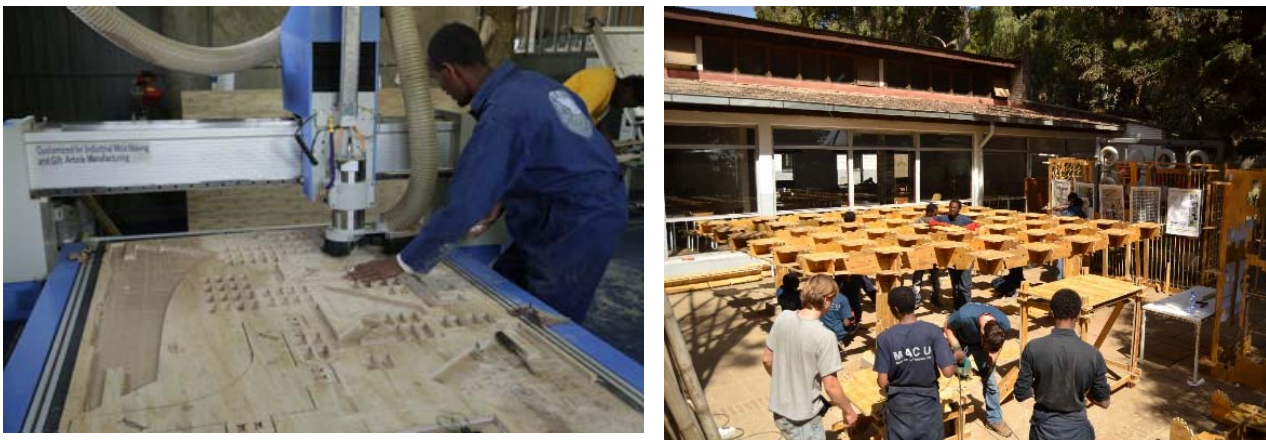
Fig. 8 MACU - CNC Milling Machine Workshop in Addis Ababa, assembling the ground floor
