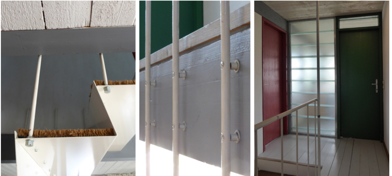
Fig.3 hanging stair of inexpensive and adjustable steel elements, screwed in glulam beams
