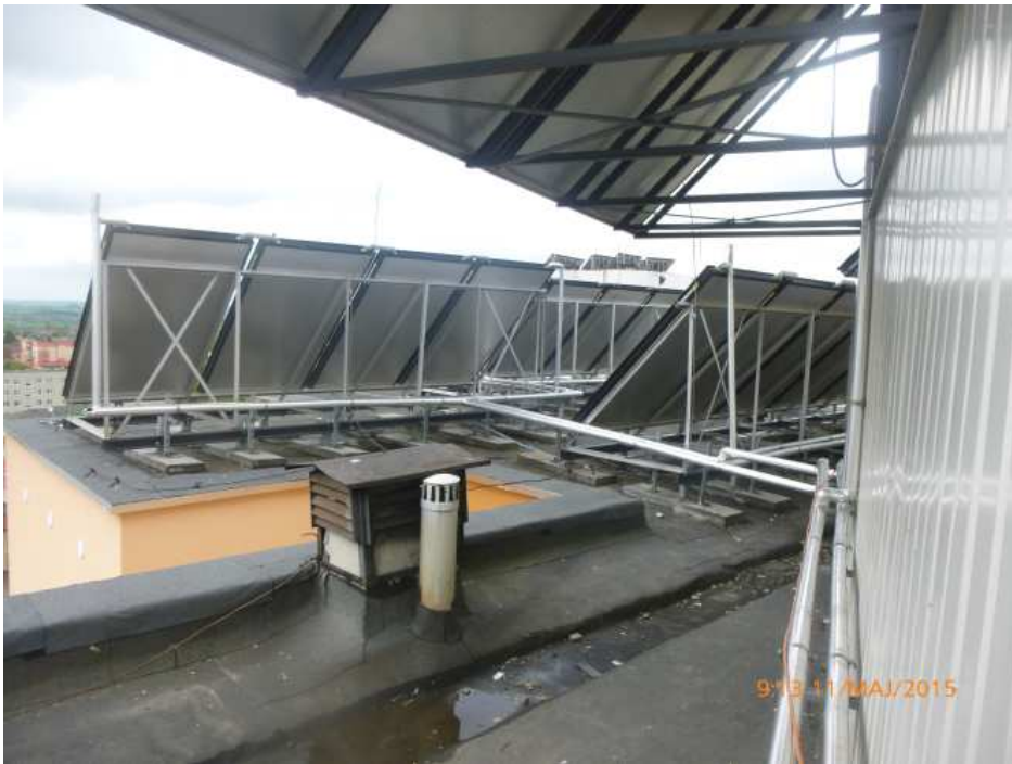
Fig. 1. Collectors on the roof of a high rised building (photo: A. Ostanska)
