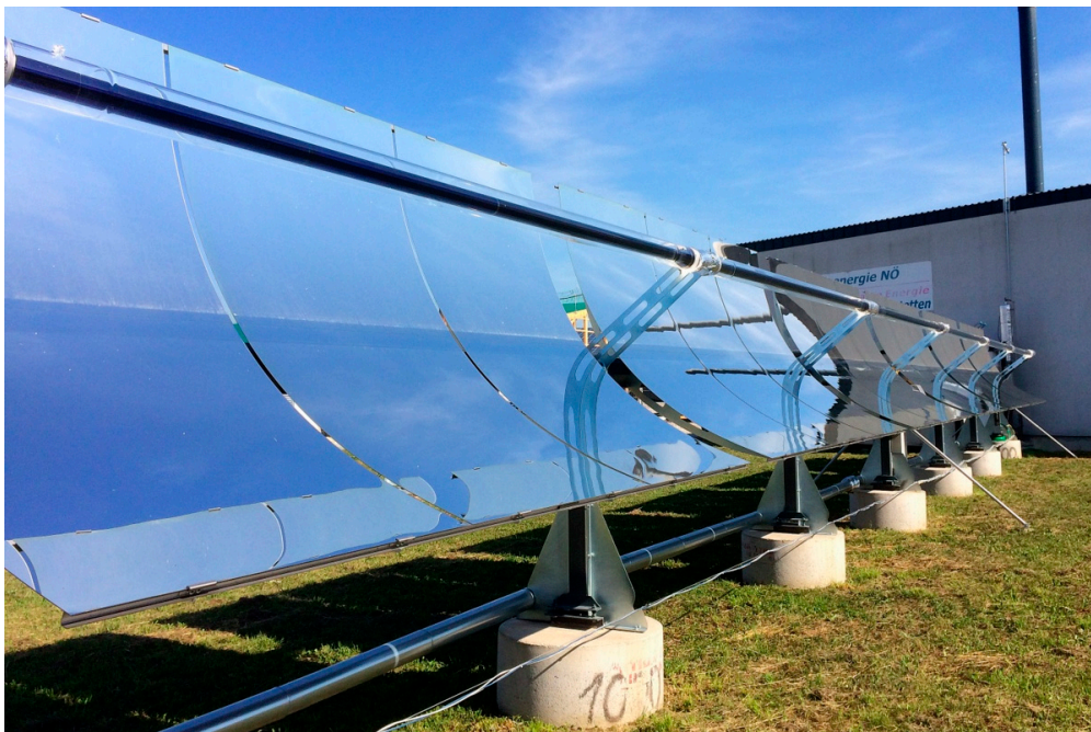
Figure 4. Solar-thermal power plant for district heating using IMK Solarmirrotec SMT-8 parabolic trough modules in Seitenstetten, Austria.
