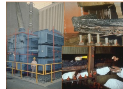
Permanent damage to the Salem New Jersey Nuclear Plant GSU Transformer (@ NASA)
