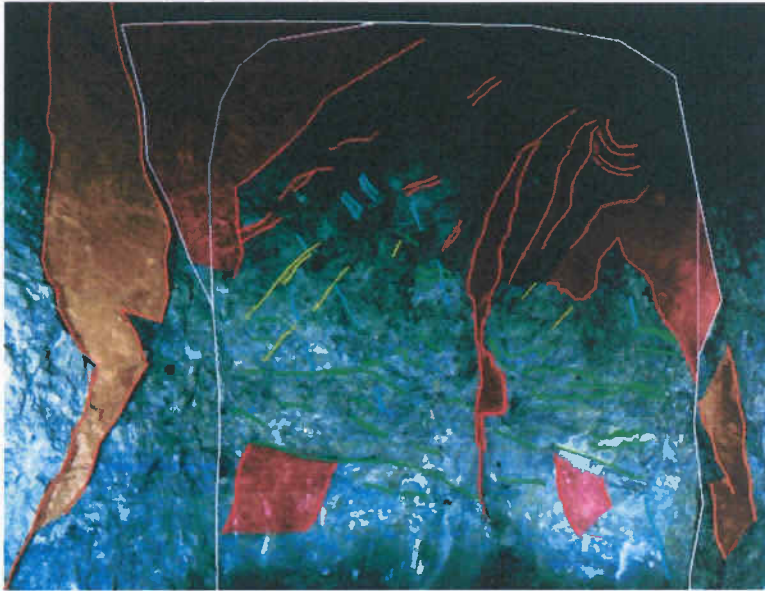
Fig. 3 Image taken in a drift tunnel in the RHI mine in Breitenau, Austria (red: fault planes, green: foliation planes, blue and yellow: joint planes, orange: fault planes in the sidewall areas, white: cross section with over break areas).
