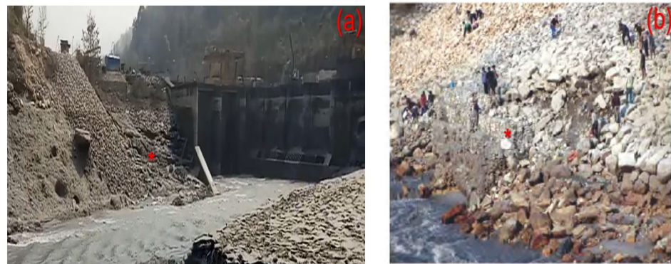
Figure 2. Instability of the slope after the draw-down is represented by (a,b) after the draw-down. * represents detail image.
