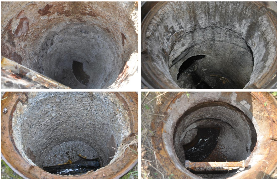
Figure 4: Examples of strongly deteriorated concrete manholes drawn to MICC.
