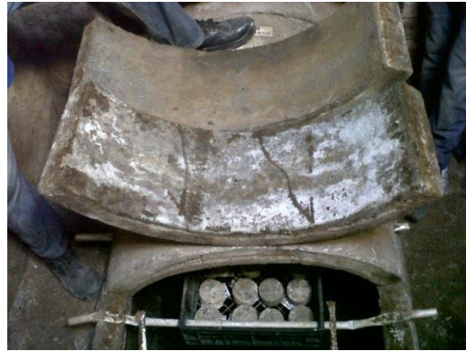
(b) Typical 'lid' samples removed for inspection and core samples suspended in the sewer
